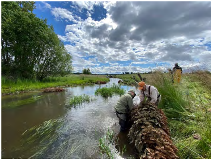
Trout Unlimited volunteers help to install Christmas Trees donated by Cornell Farms in Chicken Creek
